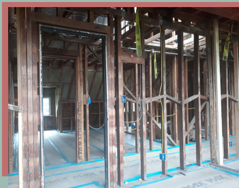
The start of construction at Kingman Hall. Photo courtesy of Steven Olesen
